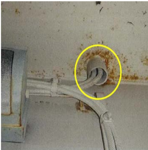
Sealing not done using fire retardant material
