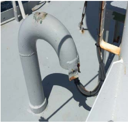
Monkey island Sealing not done using fire retardant material
